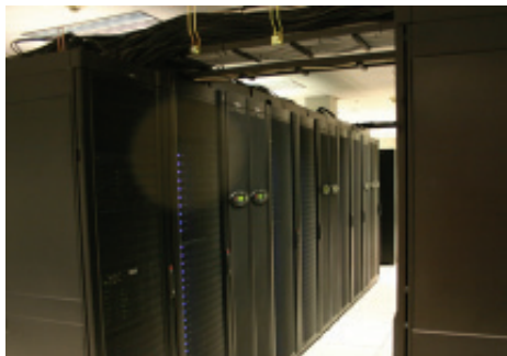
The aisle between two of Queen Bee's four rows. Note the massive amount of overhead interconnect cabling.
